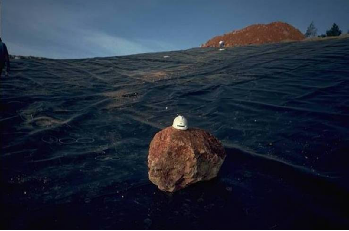
PHOTO 9 – LARGE BOULDER ROLLED ONTO GEOMEMBRANE LINER SURFACE
